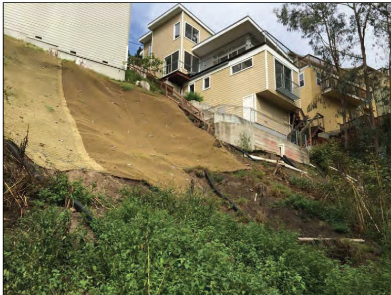
Photo 20 (Site #41): View of a hillslope failure and undermined residences upstream from Site #41. This area upslope extent of AOC 4 as discussed in the text of the report. This photo was taken from the outboard edge of the Fire Break Road upslope from the Upper Pond Legacy Road as shown on Map 2.
