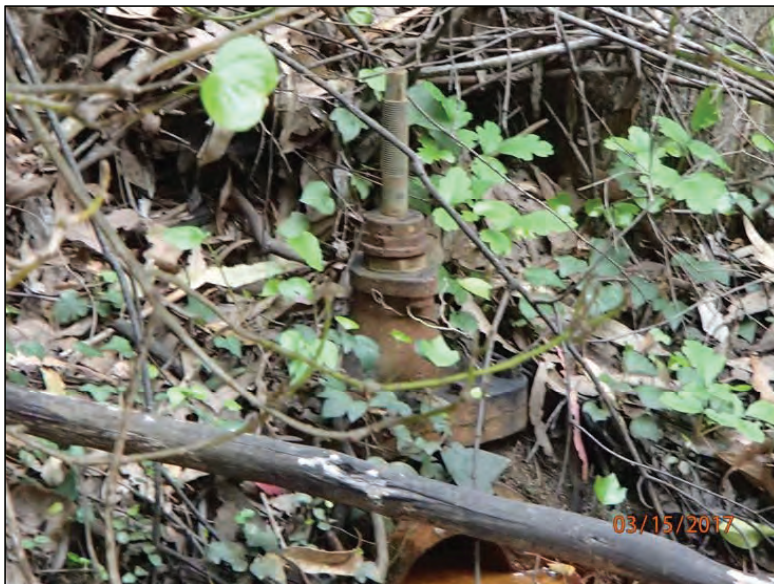
Photo 8 (Site #4): View of the seeping drainage valve at base of the dam fillslope in the axis of the valley downstream of pond.
