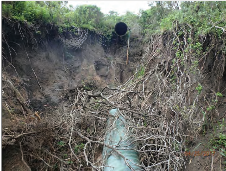
Photo 17 (Site #40): View looking upslope at the same disconnected downspout and active erosion as shown in the previous photo. The photo was taken from the base of the gully downslope of the headcut standing on top of one of the failed sections of culvert.
