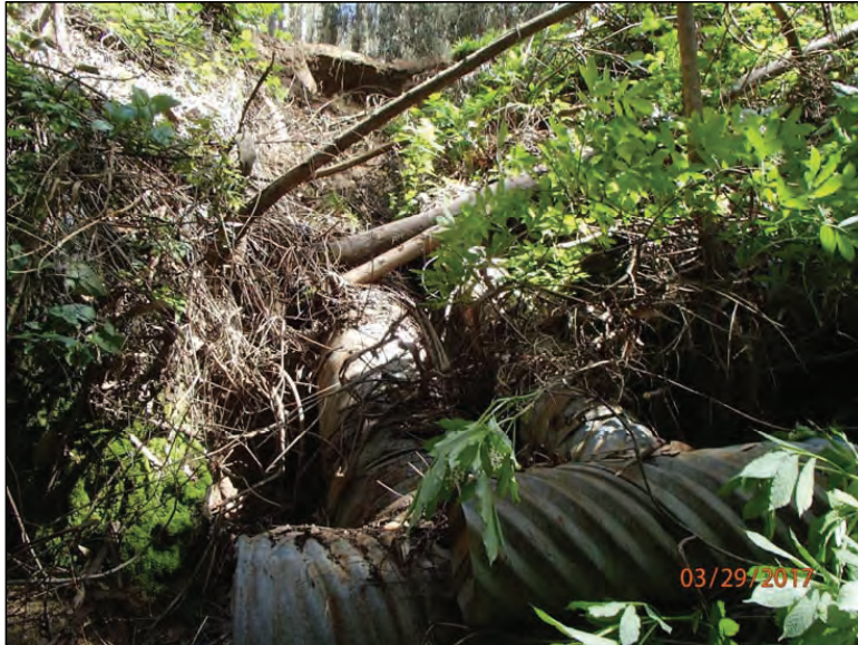
Photo 15 (Site #39): View looking upstream at the failing outboard fillslope of this plugged stream crossing. The photo was taken standing approximately 8ft downstream of the culvert outlets.
