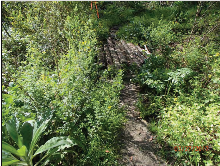
Photo 25 (Site #24): View of a makeshift foot bridge at stream crossing Site #24. The active erosion at this site is minimal, and a formal crossing should be established.
