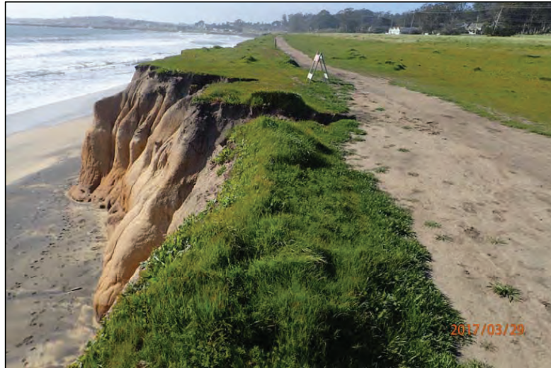
Photo 31 (Coastal Bluff Trail): View of bluff retreat looking northward along unpaved coastal trail. This photo is looking up the hydrologically connected right road reach to the gullies displayed in the previous photo.
