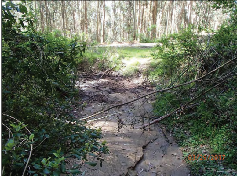
Photo 13 (Site #39): View looking downstream from the upstream extent of the of the failing stream crossing. Note the recently deposited sediments that have plugged the culvert inlets. The sediment is causing the stream flow to divert down the left road which is inducing a delivering fill failure.
