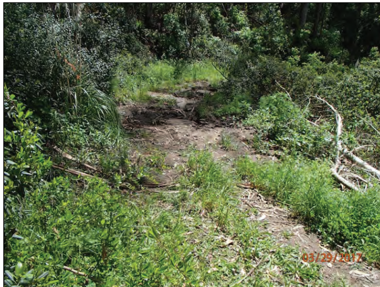
Photo 22 (Site #16): View of the fill crossing at Site #16 on the Dolphine Fire Road. Diverted stream flow is actively eroding gullies down the left road from this stream crossing.
