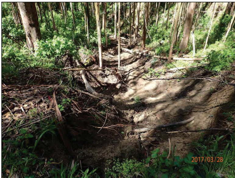
Photo 26 (Site #31): View of an outboard fill failure at Site #31 on the Vista Point Trail. Concentrated road run off had saturated the steep outboard fill and subsequently destabilized the fillslope leading to failure.
