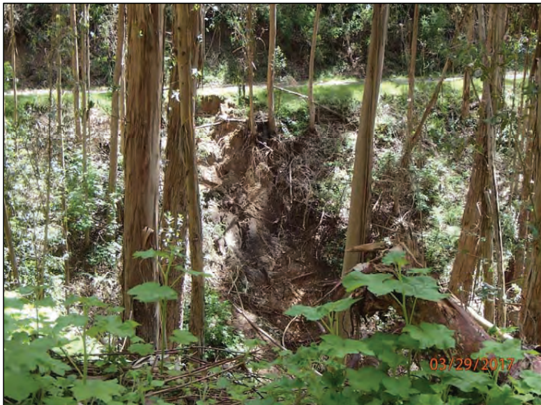
Photo 14 (Site #39): View of an outboard fill failure to the left of the stream crossing. The fill failure was induced by the diverted streamflow from the plugged stream crossing at Site #39 and excessive concentrated road surface runoff.
