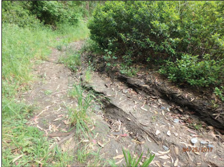
Photo 23 (Site #16): View of the left road approach to fill crossing Site #16. Diverted stream flow is actively eroding gullies down the left road from this stream crossing and delivering to a watercourse at Site #15.
