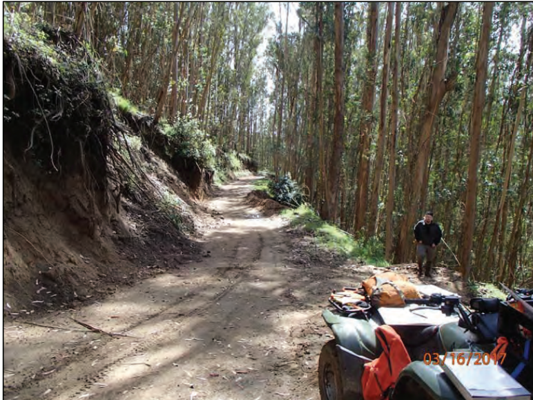
Photo 29 (Site #11): View of the hydrologically connected left road approach to landslide Site #11. Long reaches of concentrated road runoff have eroded a gully down the outboard fillslope and induced a failure.
