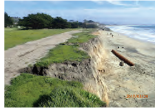
Area of concern example - bluff erosion
