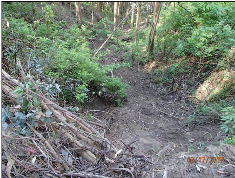
Photo 12 (Site #19): View of failing outboard fillslope, looking downslope at the fill failure deposits below the right hingeline of the fill crossing at Site #19. This photo was taken from the outboard edge of the road.
