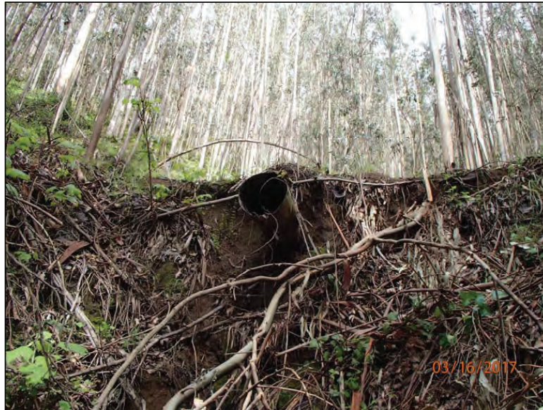
Photo 21 (Site #9): View of the perched culvert outlet at stream crossing Site #9. The culvert at this crossing is undersized and installed high and short in the fill with a 6ft drop at the outlet and subsequent outboard fill erosion.
