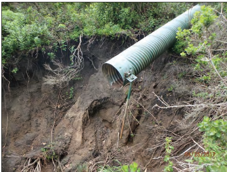
Photo 16 (Site #40): View of a section of disconnected culvert downspout at the top of an actively migrating headcut and gully below the paved Private Drive at Site #40. Oxidation exposed on the stake is indicative of the previous depth of burial prior to the episodic hillslope failure.
