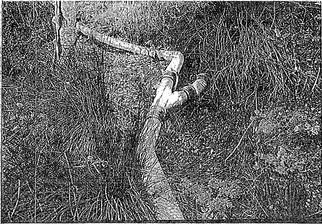
Laterals from 1306 & 1312 Bel Aire Road are connected into one 4" flex pipe
