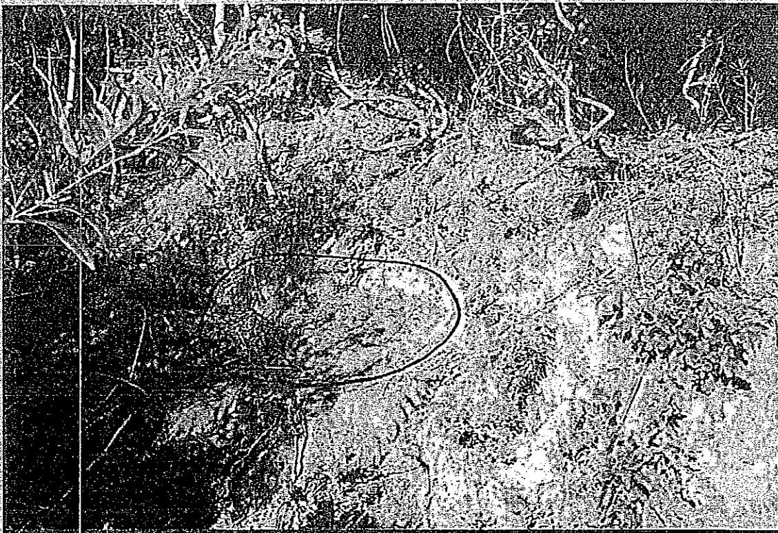
Example of MH re-exposed after being covered by sliding hillside
