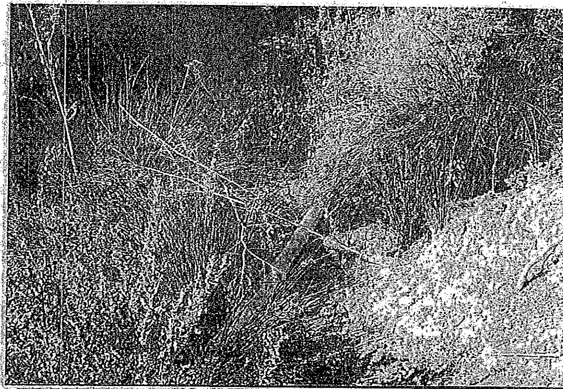
Temporary Bypass Pipe on ground between MH 11 and MH 14
