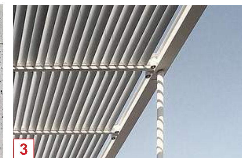
3 EXTERIOR CANOPY STEEL COLUMNS IN WHITE PAINT AND ALUMINUM TRELLIS LOUVRES IN WHITE POWDER COAT
